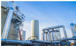
Quantum Biopower anaerobic digester plant in Southington
